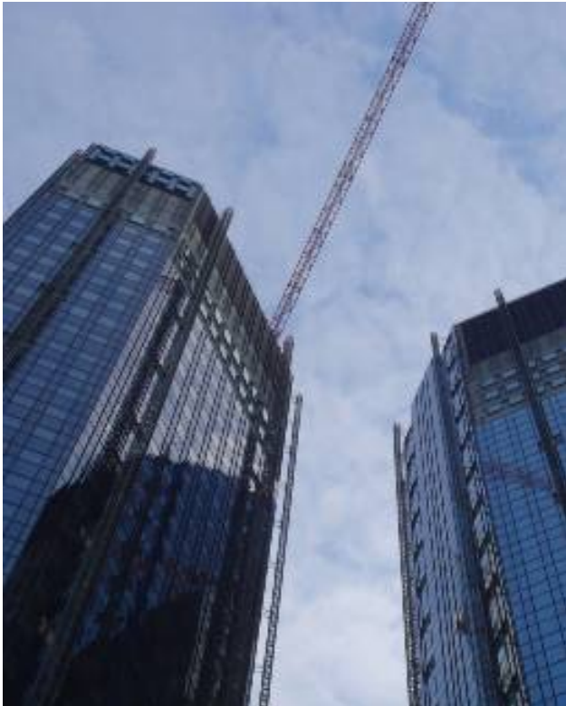
refurbishment project Deutsche Bank, Frankfurt (Main), Germany (2008-2010) source: ING. BÜRO P. BERCHTOLD
